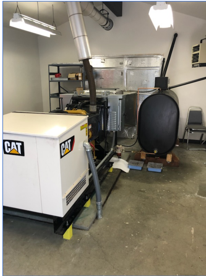
New Generator in Place at Halibut Point
